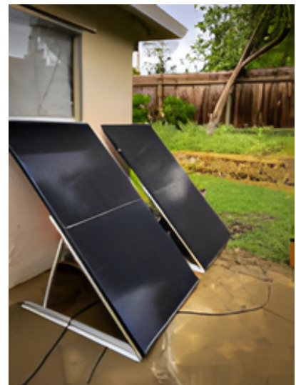
Plug-in solar array (Bright Saver)
